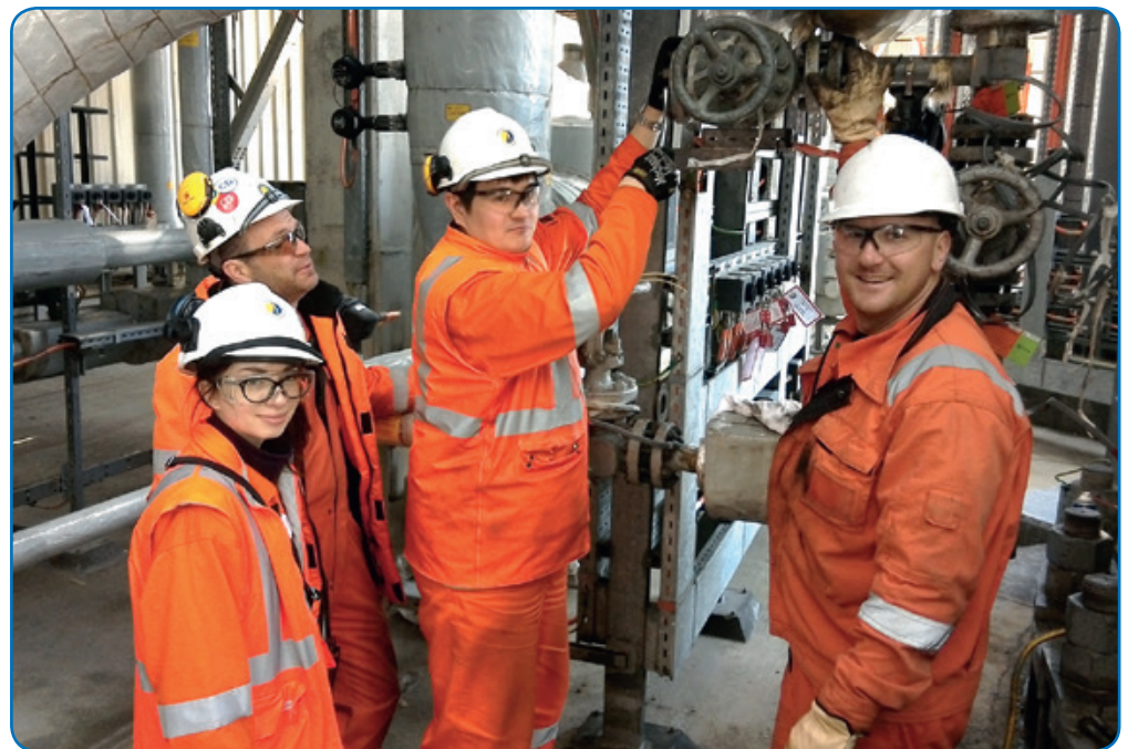
Work days. Planned technological shutdown-2020. Denis Khakimov (in the centre). In 2010, he graduated from the Ufa State Petroleum Technological University trained as an oil storage and gas and oil pipeline design and operation engineer. He has been with Sakhalin Energy since 2012
